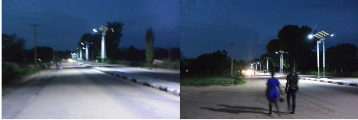
Plate 3.4: Sample of stand-alone and pole-mounted streetlights in UNIMAID campus
