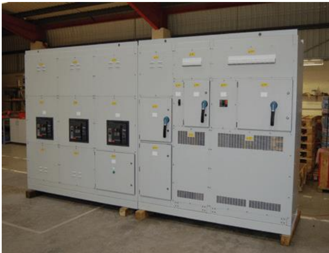
Plate 3.3: A typical low voltage switchgear cabinet Source: bourselec.co.uk/low-voltage-switchgear , 2018
