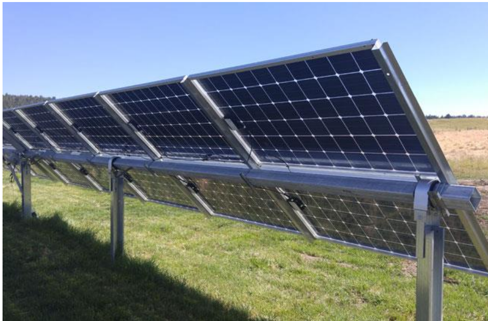
Figure 2.5: Bifacial Solar panels
