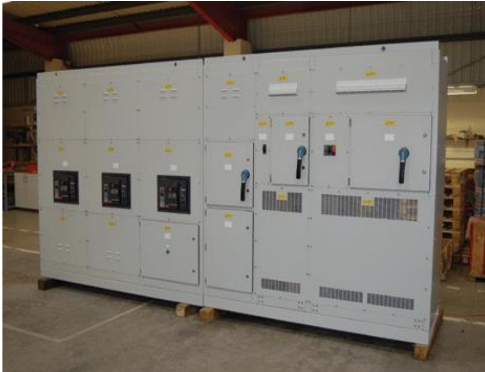
Plate 3.2: A typical low voltage switchgear cabinet
