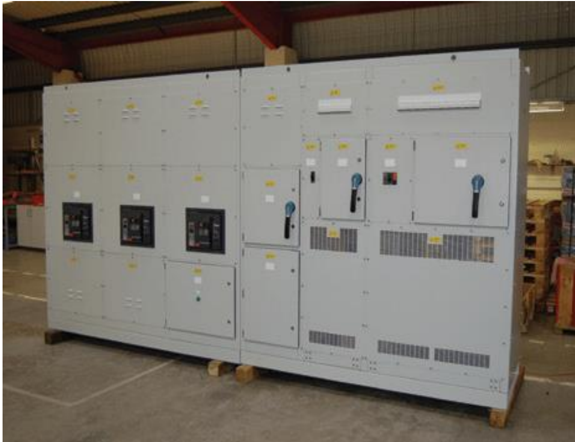
Plate 3.2: A typical low voltage switchgear cabinet
