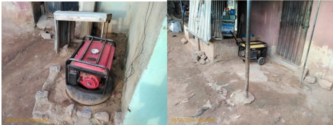
Plate 4.20: Generators used as alternative source of electricity in Mando village
