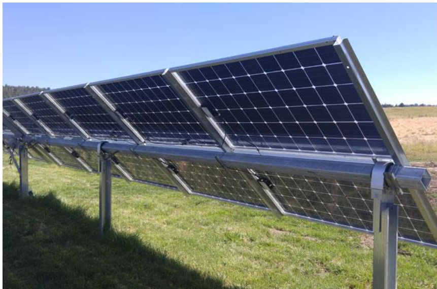
Figure 2.5: Bifacial Solar panels
