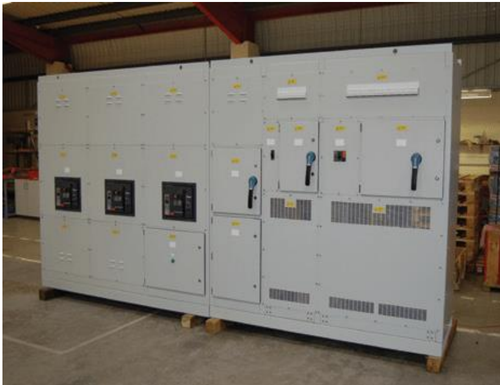
Plate 3.3: A typical low voltage switchgear cabinet
