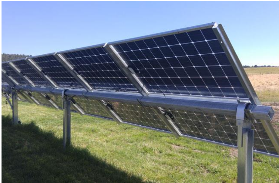
Figure 2.5: Bifacial Solar panels
