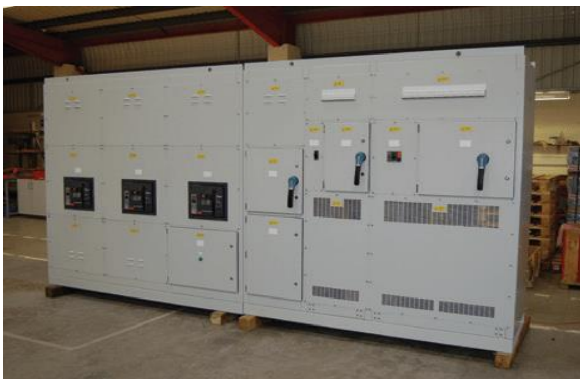
Plate 3.2: A typical low voltage switchgear cabinet
