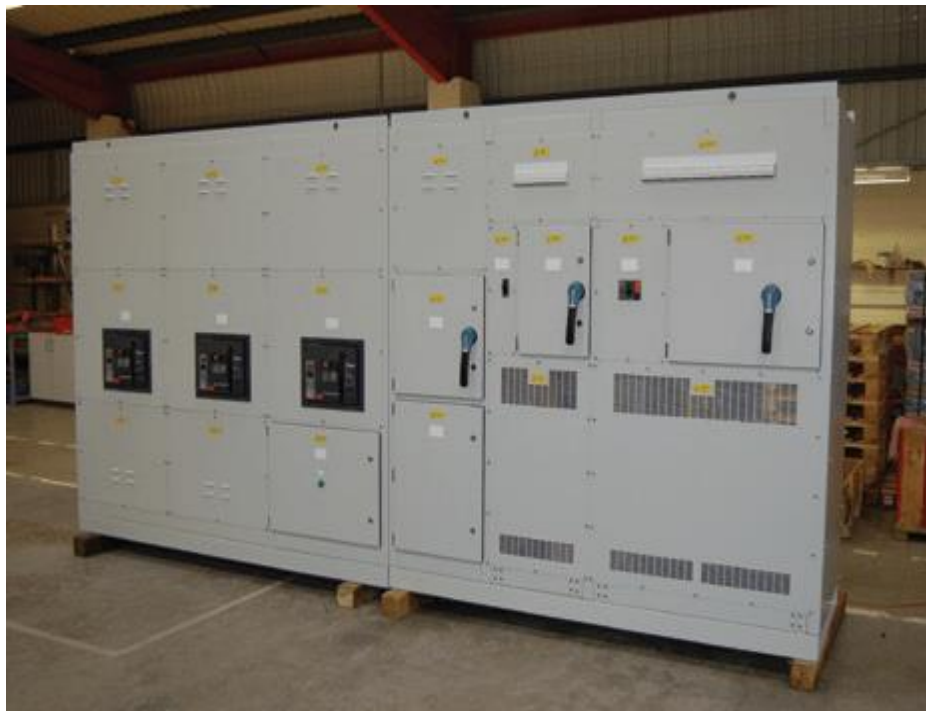
Plate 3.2: A typical low voltage switchgear cabinet
