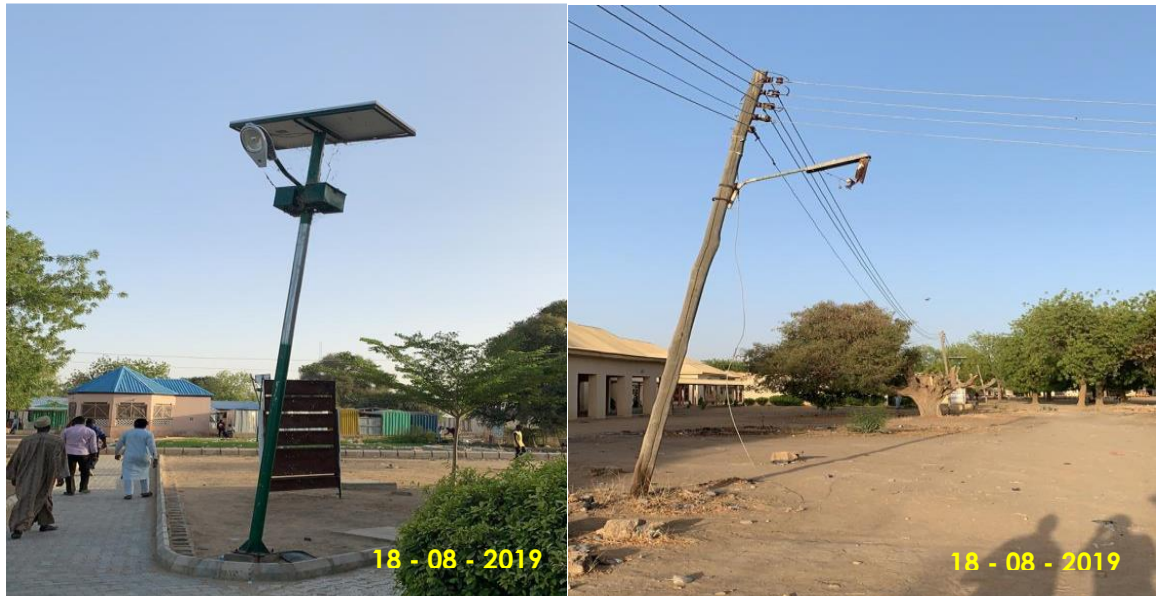
Plate 3.3: Sample of stand-alone and pole-mounted streetlights in FUGA campus
