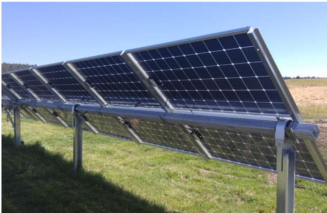
Figure 2.5: Bifacial Solar panels
